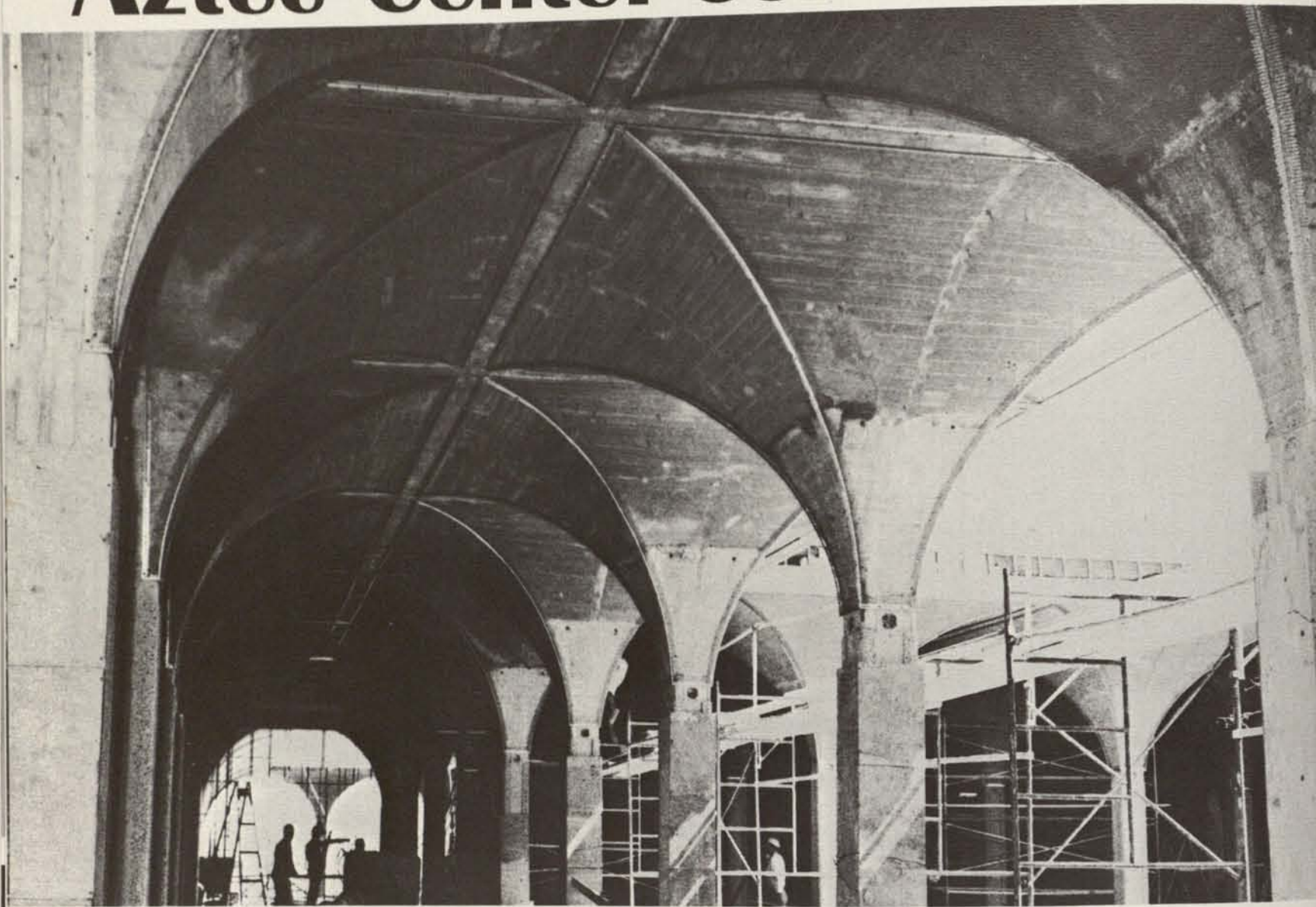
Construction had progressed to this point by early October of 1967. A view of the main level.
